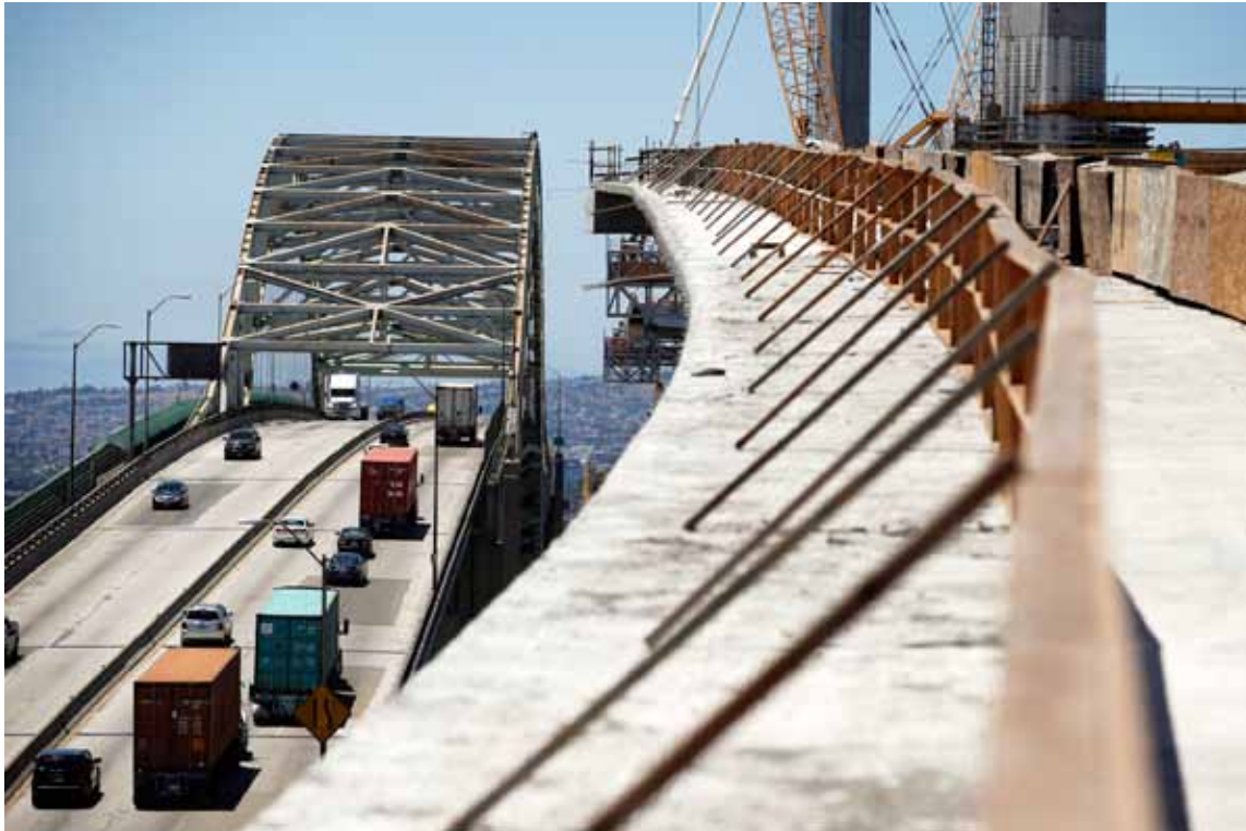
Traffic moves on the old Gerald Desmond Bridge next to its replacement bridge under construction in Long Beach, California. President Donald Trump has imposed taxes on imported steel and threatens to add auto imports to tariffs. The moves can provoke retaliatory tariffs on U.S. exports. JAE C. HONG/AP file
